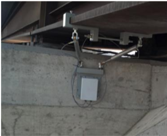
Figure 6a LVIT Mounted on Bridge
